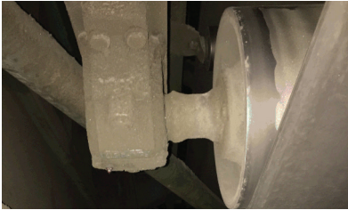
Bearing failure, Locking assembly maintenance challenges
