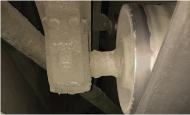
Bearing failure, Locking assembly maintenance challenges
