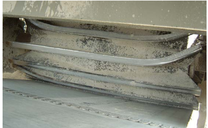
Figure 5 – Tail pulley with bent wings.
