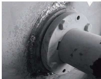
Figure 3. The hub shown here has been re-welded to the disc.
