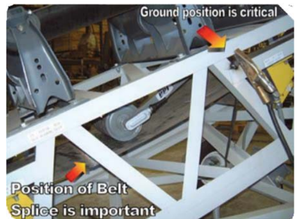
FIGURE 2.5: Permanent attachment of 3/4 inch shaft to framework. Component protection for welding has been removed for clarity.
